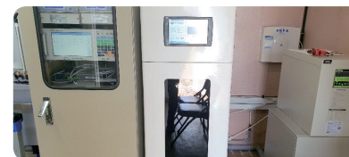
- Wastewater Treatment Plant in Daedeok Industrial Complex
