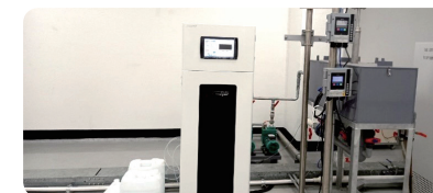
- Saemi Sewage Treatment Plant in Songsan
