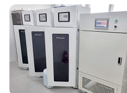
- Industrial Complex Wastewater Treatment Plant in Yongin city
