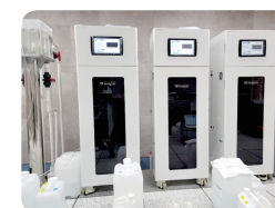
- Water Purification Plant in Geumsan
