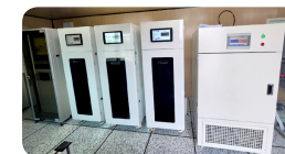
- Ganggyeong Wastewater Treatment Plant in Nonsan
