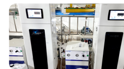
- Wolpyeong Water Purification Plant
