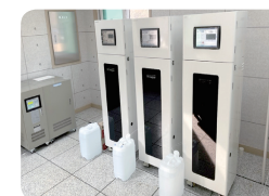
- Samcheok Water Purification Plant in K-water
